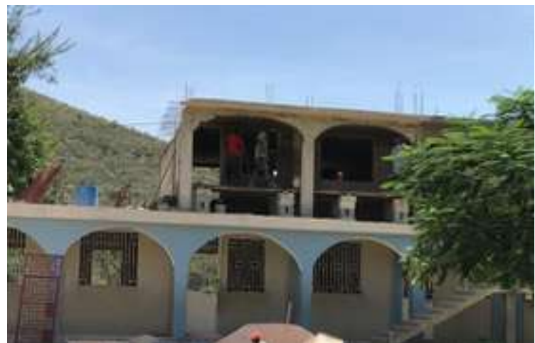
Ready to top it off! imagine a new classroom on the second floor, to the left of the two rooms already there.
